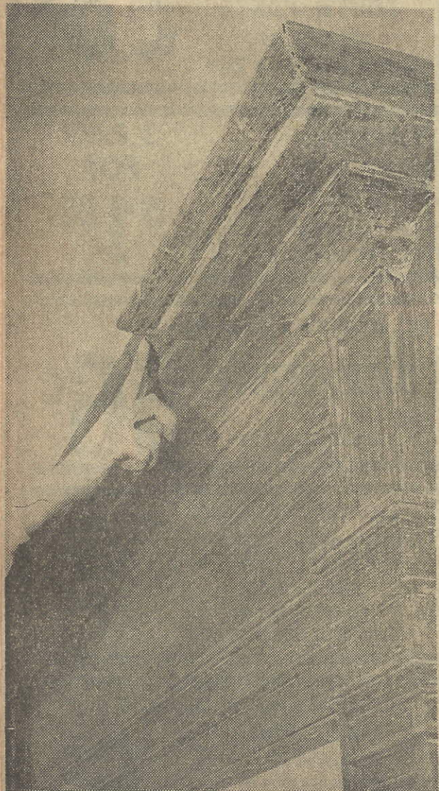
MANTEL PIECES in the bed chambers of Ainsley Hall Mansion are wider at the corners to accommodate the candle holders which were once used there and to keep the candle flame away from the wall.
