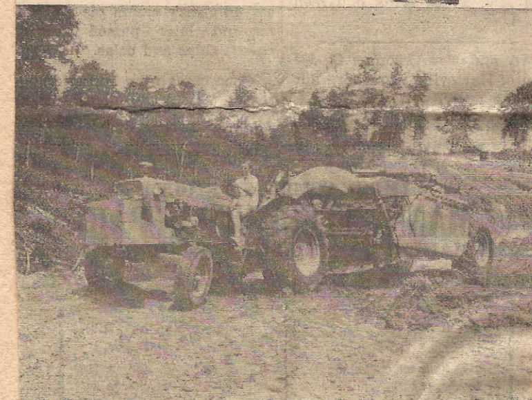
POND CONSTRUCTION — Mrs. L. L. Miller assisting her husband with pond construction on John L. Pope, Jr., farm. Mrs. Miller is operating a self-loading pan while her husband runs the bull dozer.
