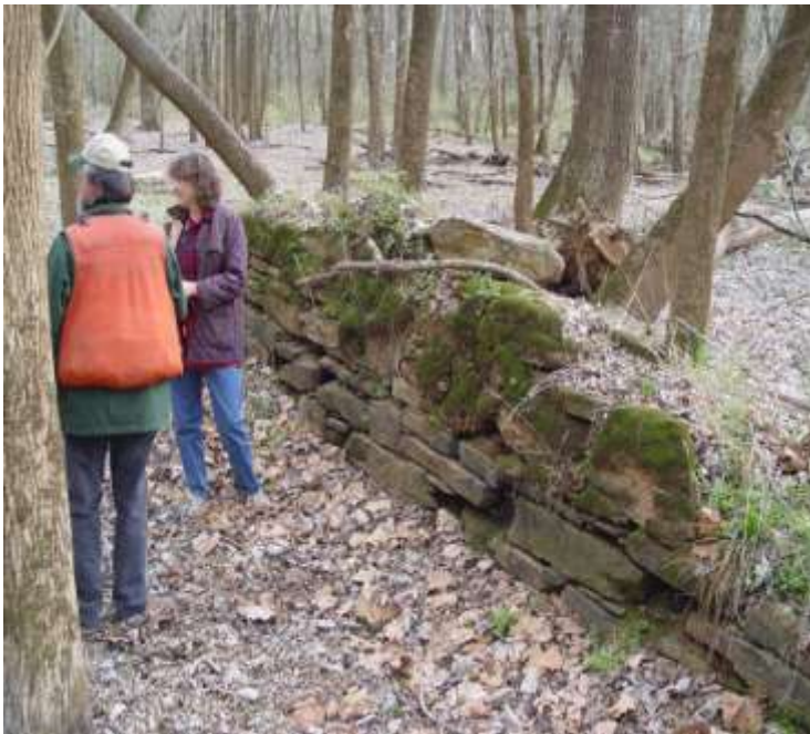
Segment of diversion canal wall Archaeologist Mike Harmon (left), Pelham Lyles (right)
